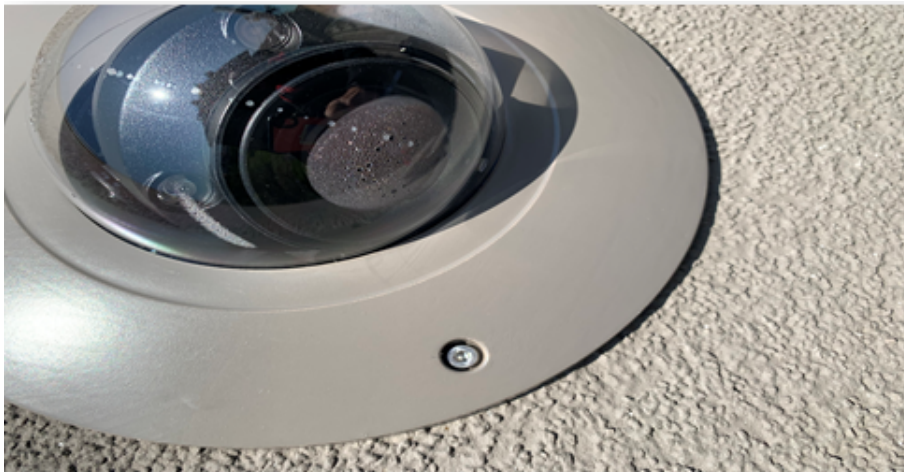
Figure 1-1 Moisture inside the camera
